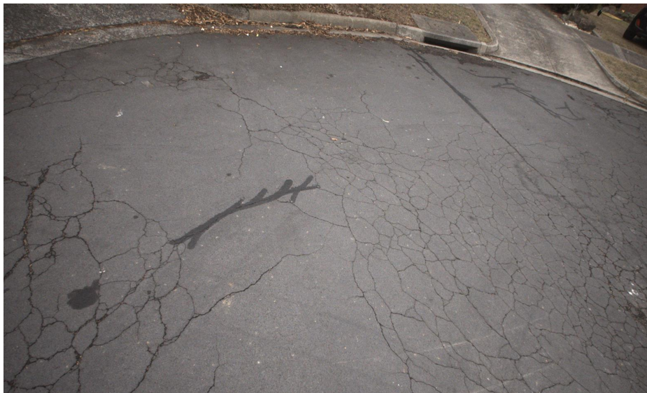
Figure 4 Snapshot of a very poor road surface (Wallmah Close in Templestowe)
