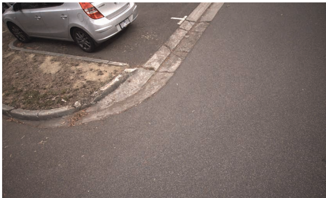
Figure 21 Snapshot of a very poor Kerb and channel in Anderson Park off-street carpark.
