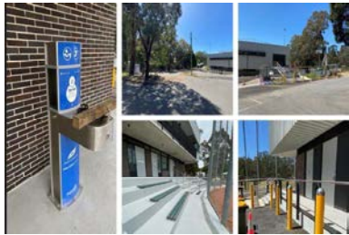
Deep Creek Reserve Pavilion new foundation, posts, retaining wall, path, synthetic grass and shed
