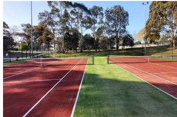
Park Orchards Tennis Club Courts synthetic resurfacing, new fencing, and net posts/nets
