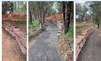
Jumping Creek Road Reached detailed design stage, with recreational trail works in progress
